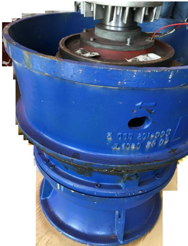
Picture of Existing Pump (Lower)
