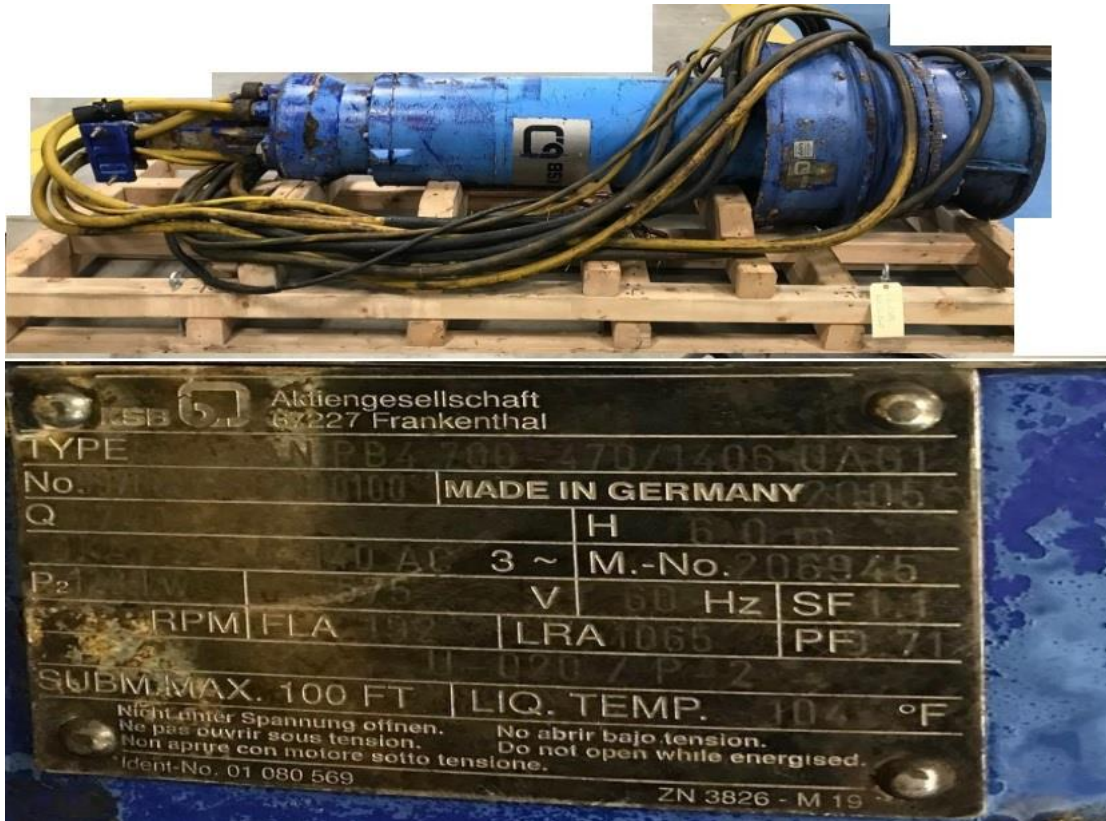
Picture of Existing UV Pump and Nameplate
